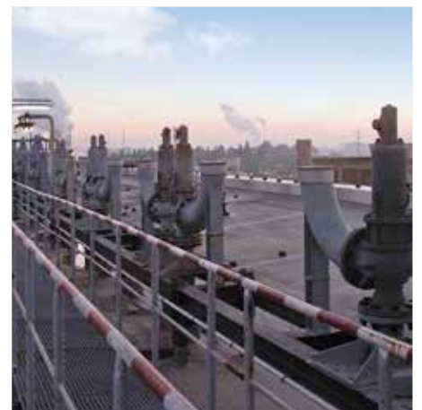
IMI Bopp & Reuther high-pressure safety valves type Si 63 installed
