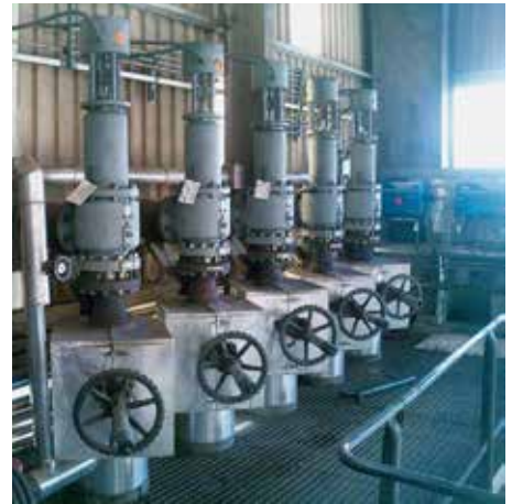
PC 50 control unit with connected pneumatic assisted springloaded safety relief valve
